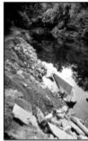
Restoration of this section of bank on Pennypack Creek was started in 1998 to control bank erosion.
